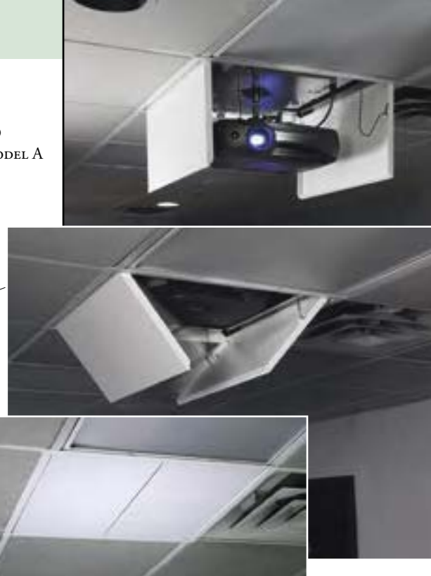
LCD Lift Model A with standard bomb bay closure located at Manitowoc Beverage Equipment, Sellersburg, IN. Installation by ISSG and photography by Kenneth Hayden, both of Louisville, KY.
