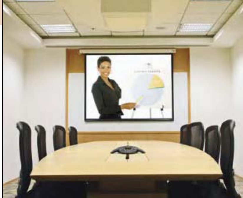
Baronet installation at World Bank (New Delhi) India. Architect: Raj Rewal Associates, New Delhi. Photo courtesy of the project system integrator: Total Presentation Devices, New Delhi.
