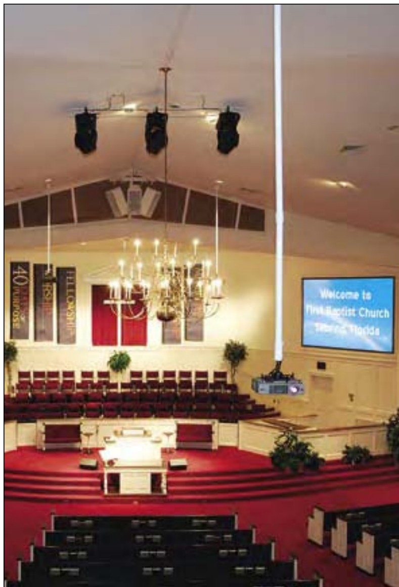
(Left) Three Accuset mounts field painted white. Location: First Baptist Church of Sebring, Florida. Design/Installation: Bassett Electronics, Inc., Sebring. Photography: © 2005 Kent Smith, Charlotte, NC.
