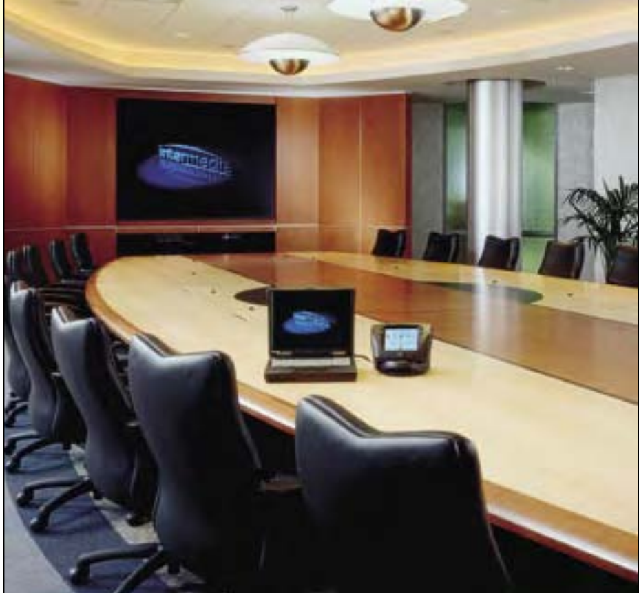
DiamondScreen installation at Intermedia/Worldcom. Dealer: Audio Visual Innovations. Photography: © 2001 Chroma Inc. All located in Tampa, Florida.
